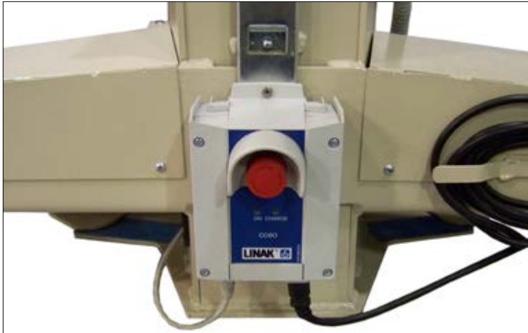
Red Emergency Power-Off Button
